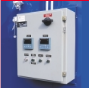
U.L Listed Flame Control Panel
